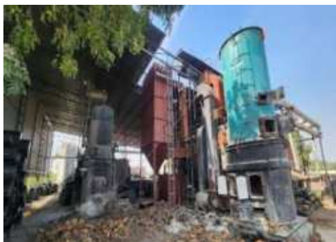
Thermic Fluid Heater
